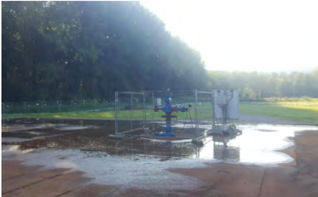
Figure 18-4 Steig-1 well head (suspended as a potential producer)
